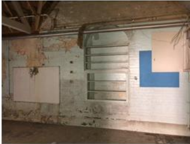
School interior to party wall with house. Note oil feed pipe running full length of school to oil tank in rear garden. (Oil tank to be drained and demolished.)
