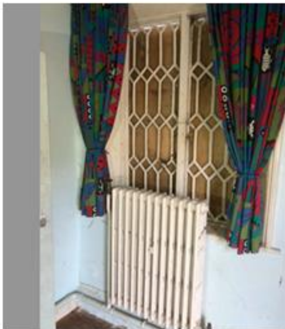
Only existing one of three original cast iron lozenge design front windows to front façade. Replacement required for original two missing windows to match existing for Grade 11 building.
